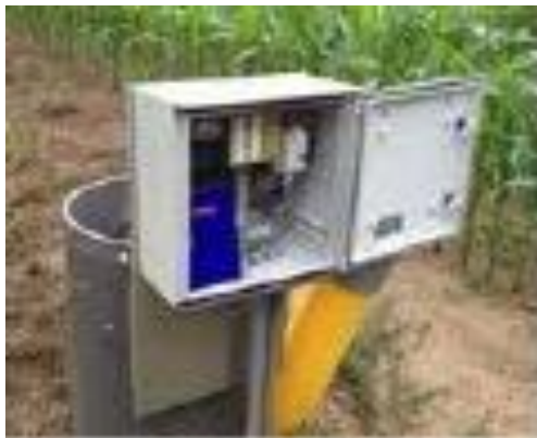
Figuur 4. Installation for Climate Adaptive Drainage (CAD). (Source: STOWA 2012-33).
