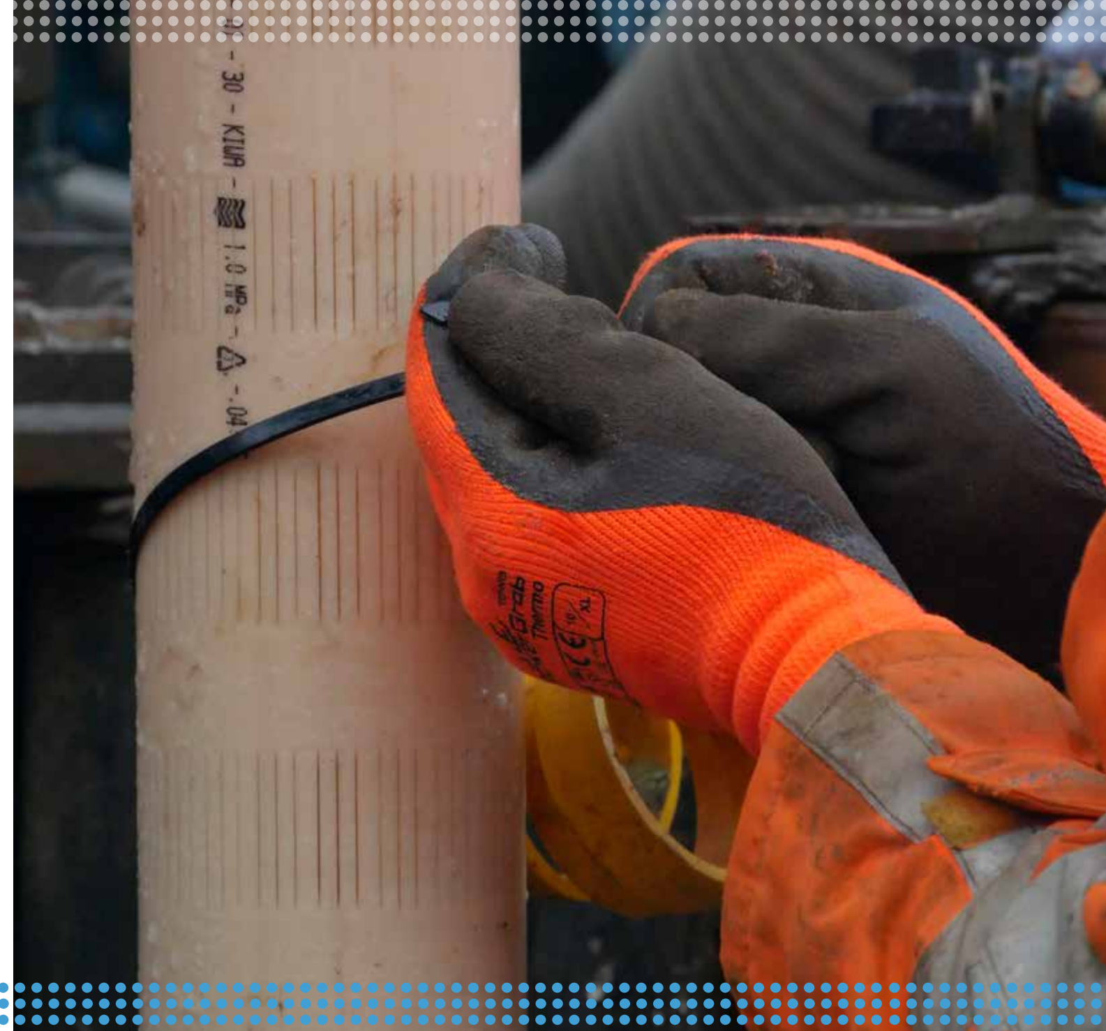
The vertical infiltration pipe
