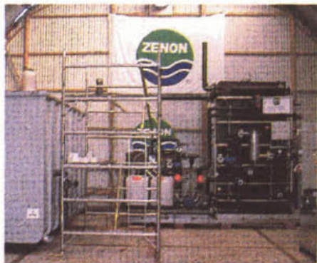
Figure 74 - Photograph Zenon pilot plant
