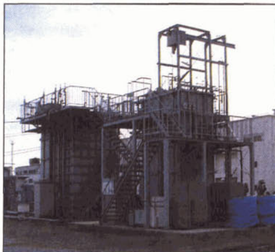
Figure 11 - MBR pilot in Misato Japan (Mitsubishi)
