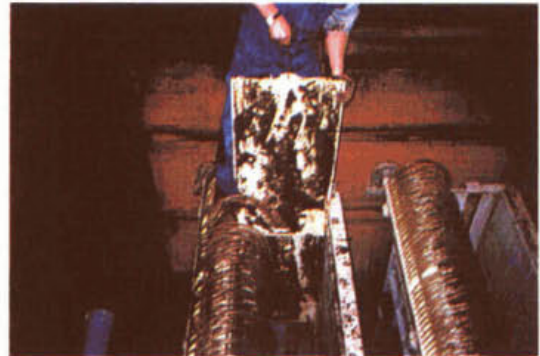
Figure 9 - Sludge on the membranes due to an operational error
