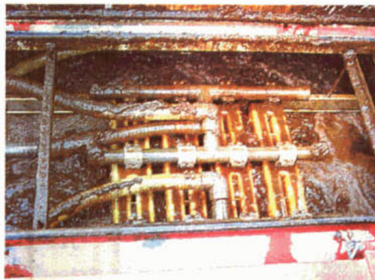
Figure 3 - An industrial MBR where chalk scaling predominates and is controlled
