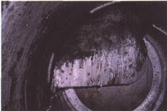
Figure 14 - Accumulation of screenings
