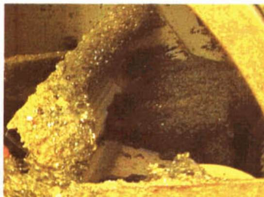
Figure 17 - Accumulation of screenings
