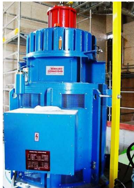
Figure 4: Alternator in Seine Aval WWTP (Nitrification Unit)
