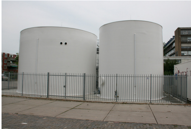
FIGUUR 2.4 MBR TANK (L) EN VERGISTER (R)
