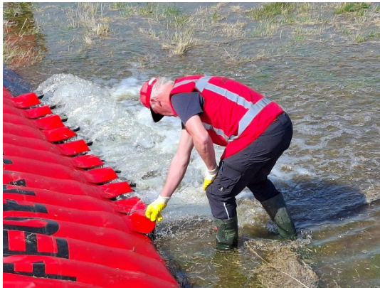
Figure 2.84 To accelerate the release of the water retained by the BFW, the discharge openings incorporated into the barrier were opened by pulling apart the hook-and-loop fastener seals.
