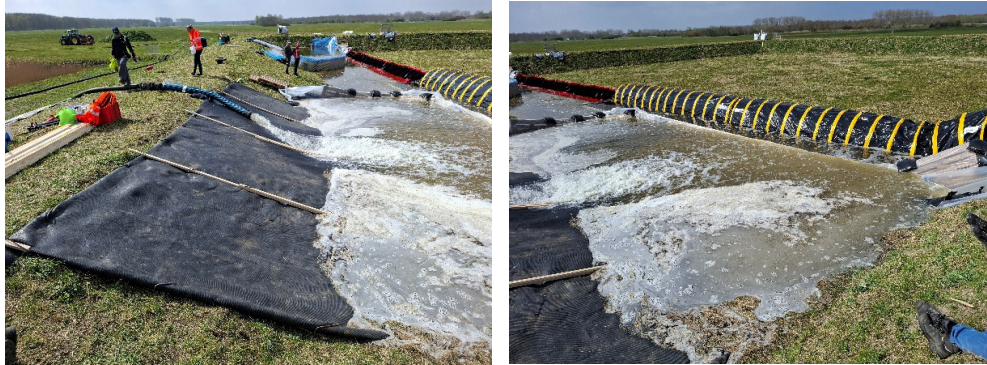
Figure 2.31 The basin is filled further until the overtopping flow from the Euro pallet structure also fills the space between the Euro pallet barrier and the TubeBarrier located behind it. The water then enters the TubeBarrier through the openings on its water-retaining side, resulting in the filling of the tube.
