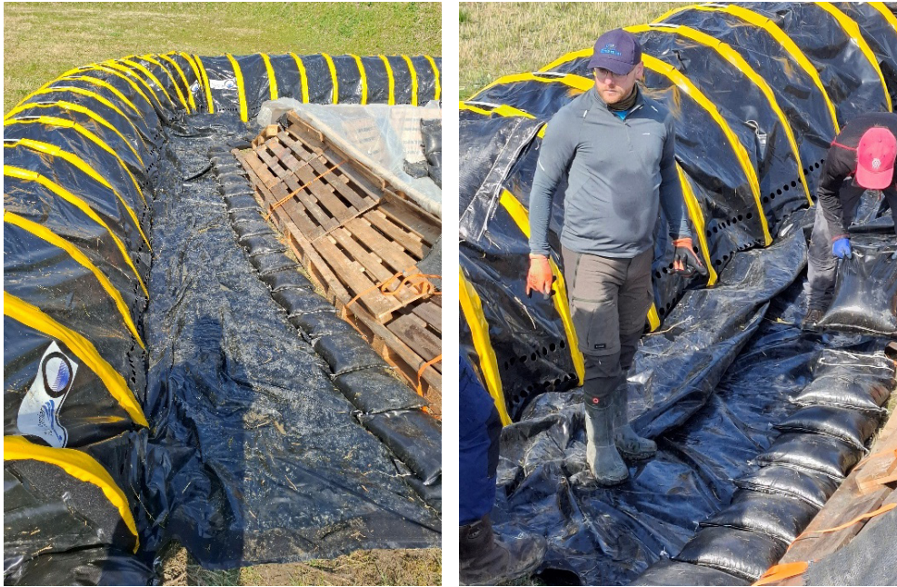
Figure 2.43 The highly irregular contact between the sheeting and the grass-covered ground surface is clearly visible, which may adversely affect the watertightness of the barrier.
