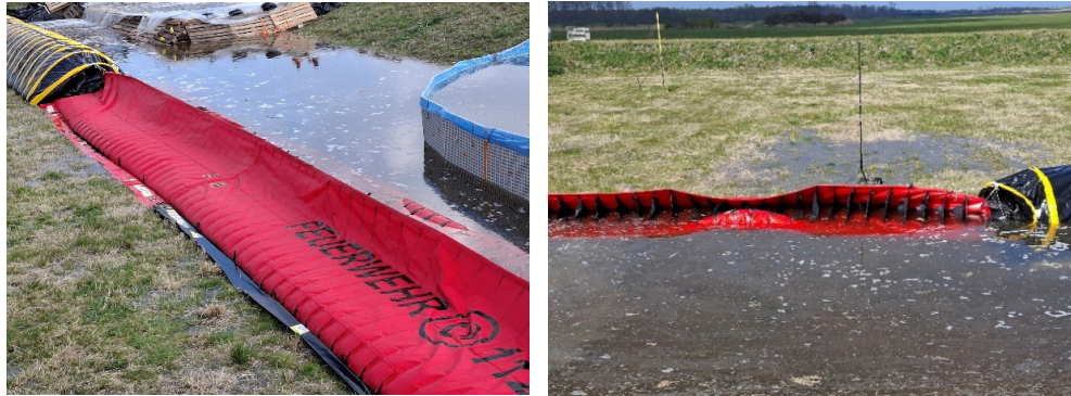
Figure 2.80 On the landward side of the BFW, leakage is observed as a result of underseepage beneath the barrier. Because the waterside edge of the membrane was not ballasted with sandbags, the membrane partially lifted under hydraulic loading, allowing water to pass beneath the system.
