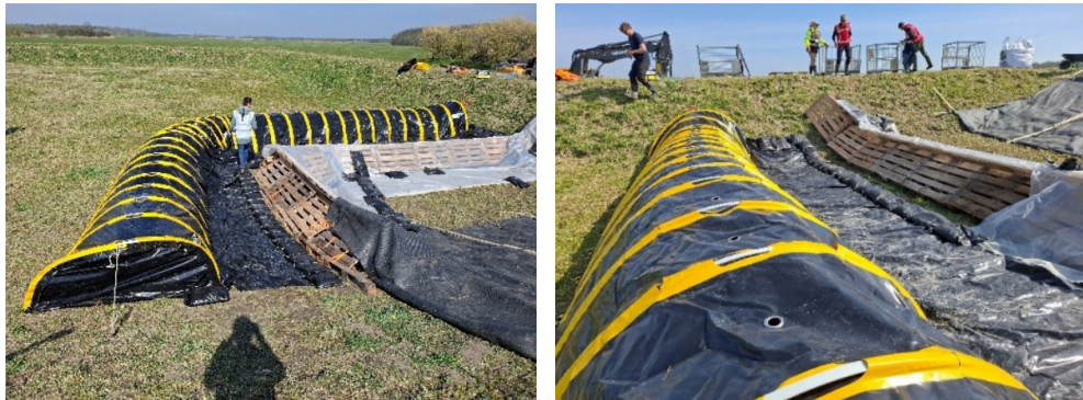
Figure 2.42 The TubeBarrier skirt was deployed, but owing to the limited space available relative to the Euro pallet barrier, it could not be laid flat on the ground surface and consequently contained multiple folds. The outer edge of the skirt was weighted down with sandbags to mitigate underseepage beneath the barrier.
