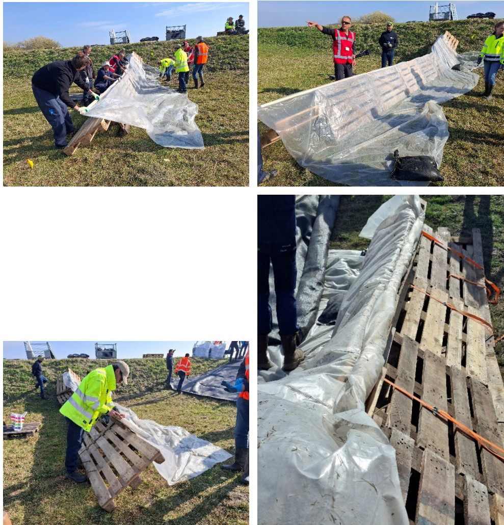
Figure 2.26 The timber battens have been rolled into the plastic sheeting in the wrong direction at the top of the Euro pallet structure, creating a depression in which overtopping water can accumulate.
