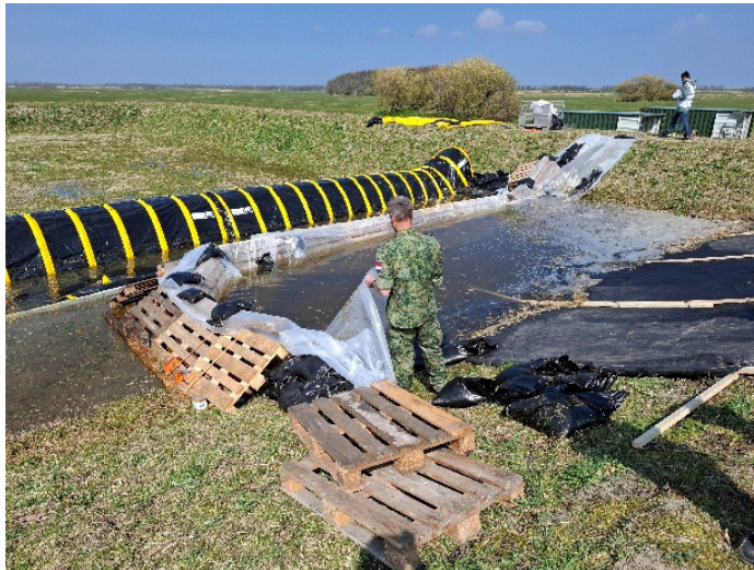
Figure 2.32 The Euro pallet basin after cessation of the water supply. The water level in the basin gradually decreased over time due to a combination of underseepage beneath the barrier and leakage through the plastic sheeting.
