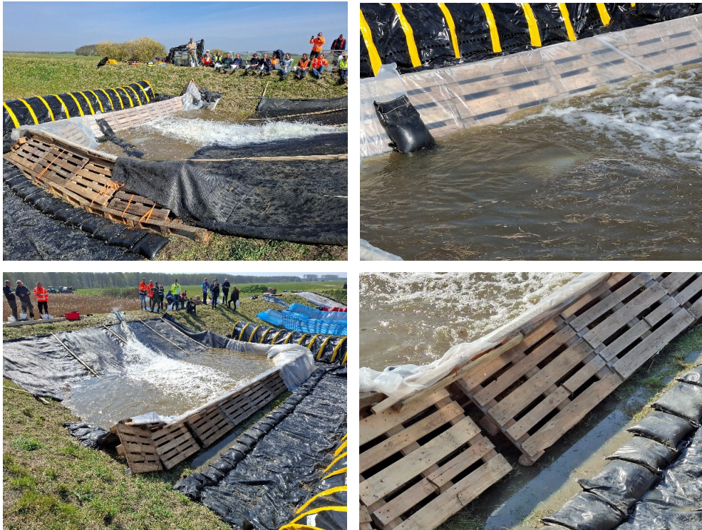
Figure 2.33 Test of the Euro pallet barrier on the second day of the exercise. Compared with the first day, the barrier showed improved watertightness and reduced leakage.
