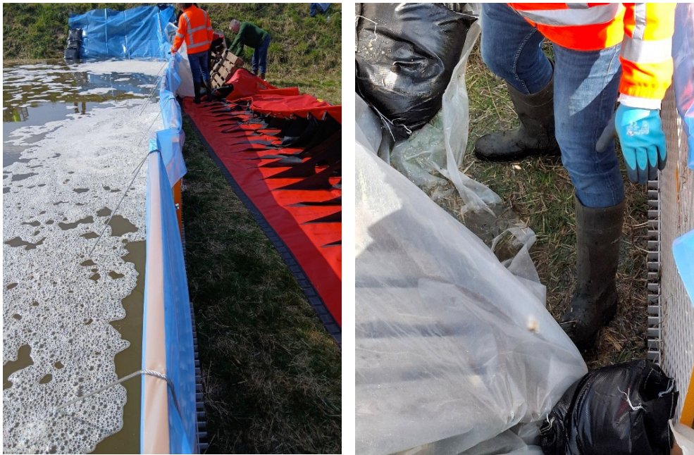
Figure 2.60 The basin has not yet reached its full design water level. Nevertheless, underseepage is already evident at the lateral transitions between the barrier and the embankment slopes.
