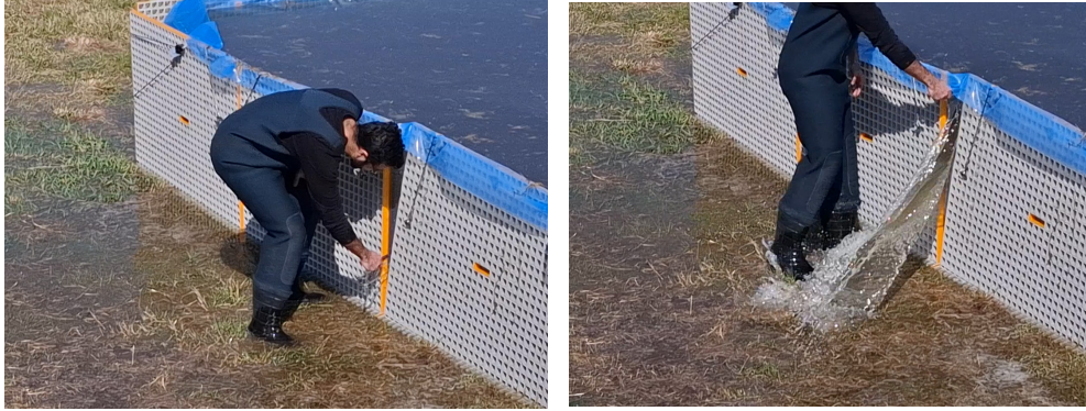
Figure 2.70 The tear extended over approximately two-thirds of the barrier height.
